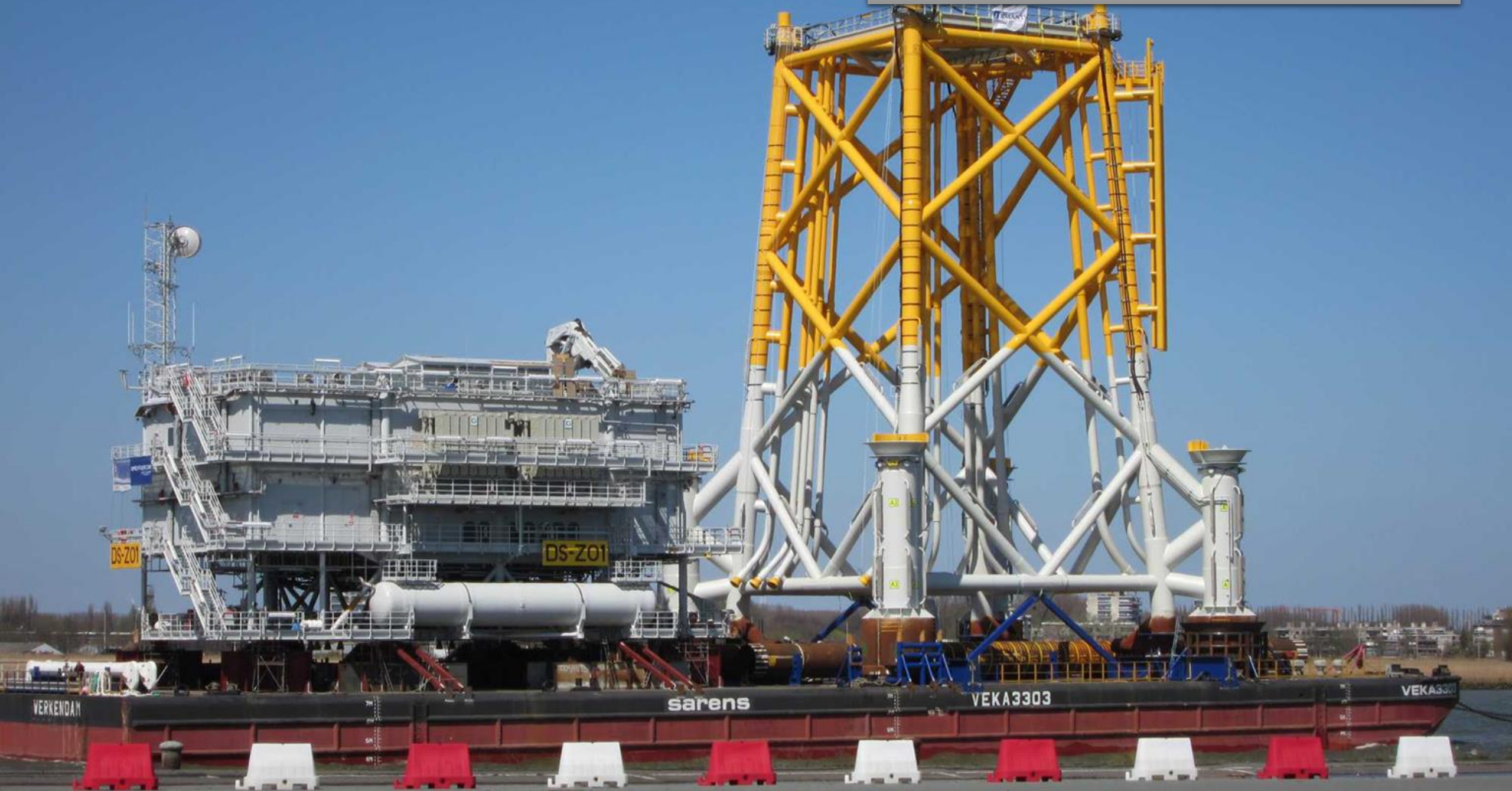
Offshore Wind Farm, West of Duddon Sands
